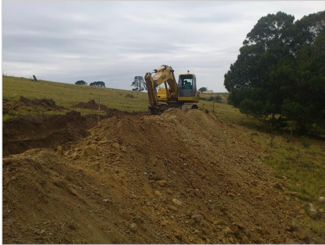
Image F: Depicts machinery used to dig ditches in preparation for infrastructural provision (Aurecon, 06/07/2012).
