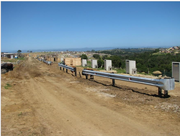
Image K: Depicts the width of road provision planned for serviced sites (Aurecon, 11/28/2013).
