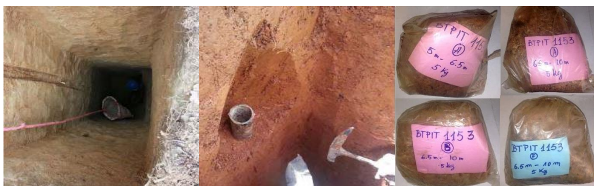
Figure 3.3 Pit excavation showing pit sampling procedure, manual techniques and samples received (A1 (5 – 6.5 m), A2, B and F (all 6.5 – 10 m)) (Desharnais et al. , 2014)
