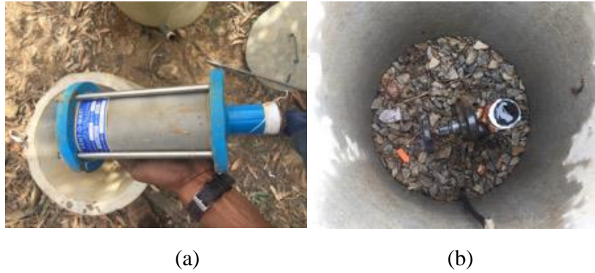
Figure 5-49: (a) Air valve (b) BS 8 Pipeline stop valve connection
