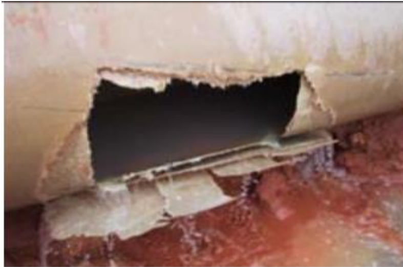
Figure 2-50: GRP pipe failure (Australia, 2003)
