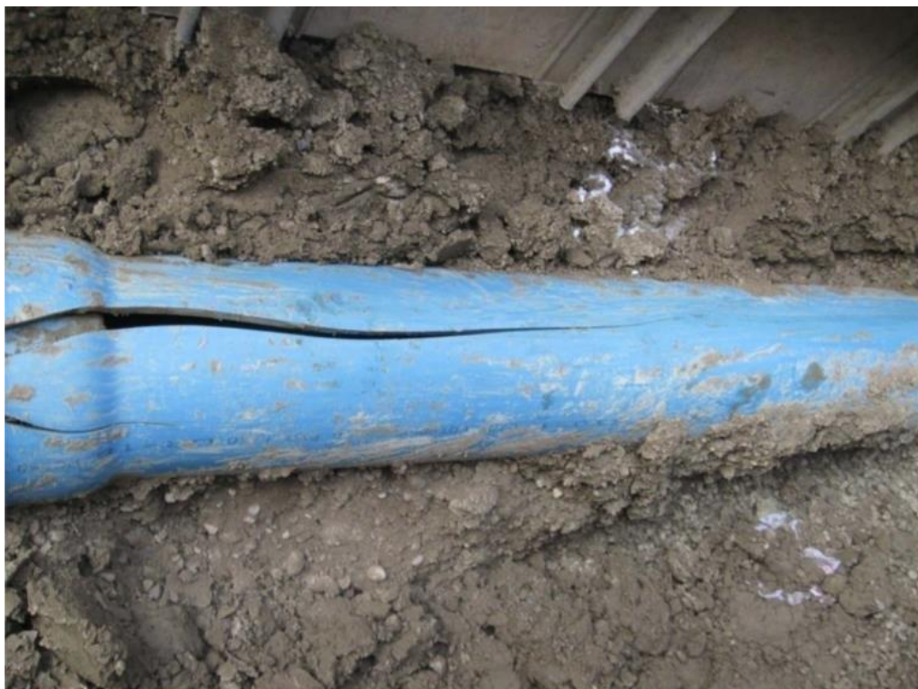
Figure 2-43: PVC pipe failure (Dueck, 2010)
