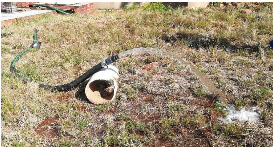
Figure 5-13: Constant flow observed after valve AV1 was closed
