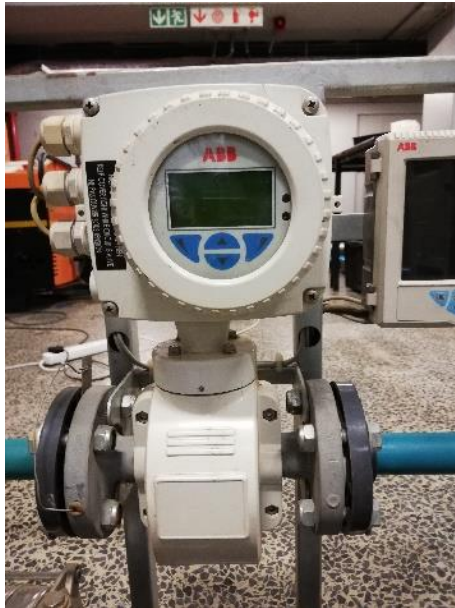
Figure 4-8: Electromagnetic flow meter display panel
