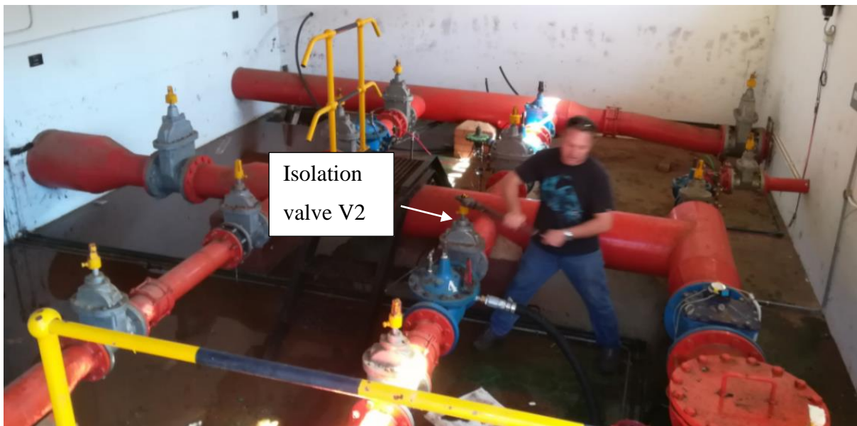
Figure 5-35: Carina street inside chamber housing isolation valve V2
