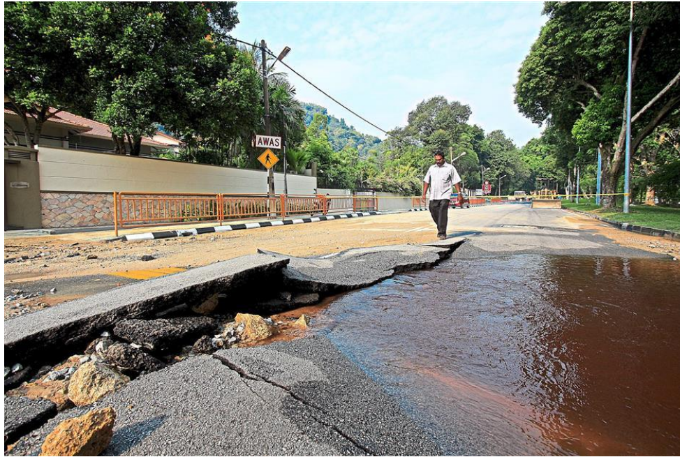
Figure 2-2: Road damage caused by underground undetected leak in Tanjung Bungah, Penang (Ying, 2015)
