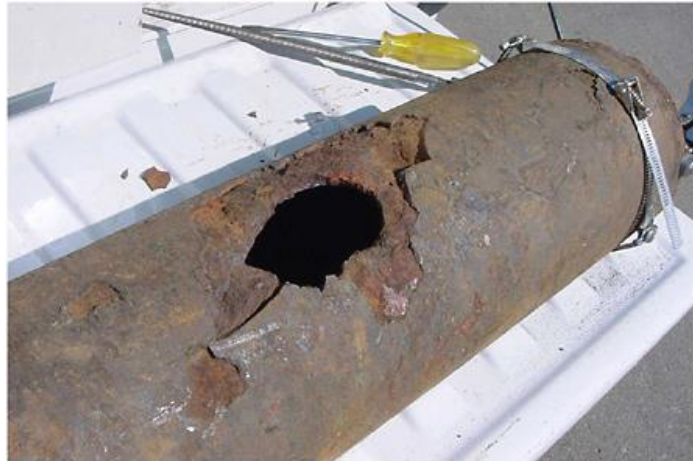
Figure 2-31: A failed cast iron pipe (The National Academies of Science and Engineering, 2011)
