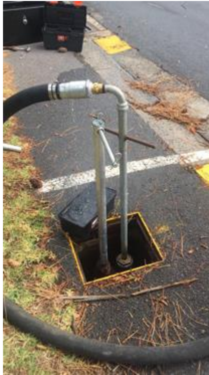
Figure 6-17: The underground fire hydrant connection
