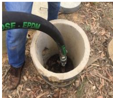
Figure 5-50: PCAE connected to the BS 8 pipeline
