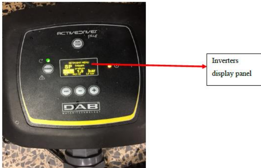
Figure 4-7: Inverter showing a set point pressure of 1 bar
