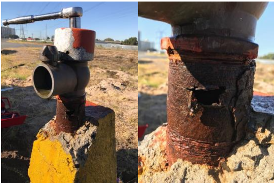
Figure 5-82: Failed fire hydrant pipe
