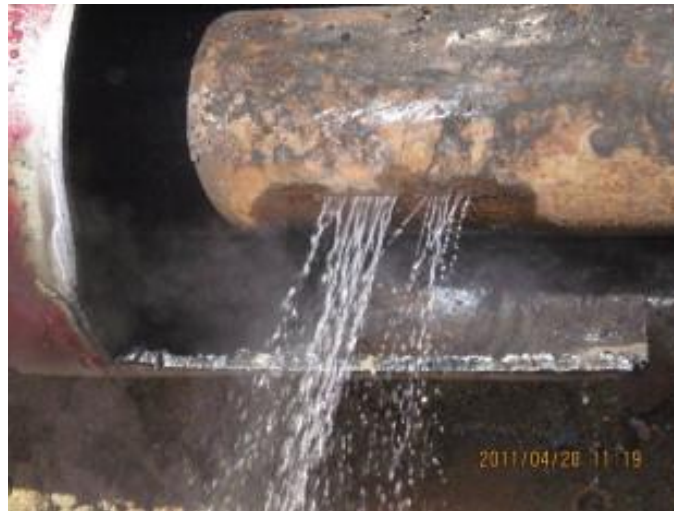
Figure 2-40: Photograph of a failed weldment in a steel pipe (Lee et al., 2013)
