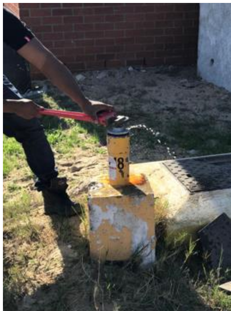
Figure 5-85: Covered fire hydrant
