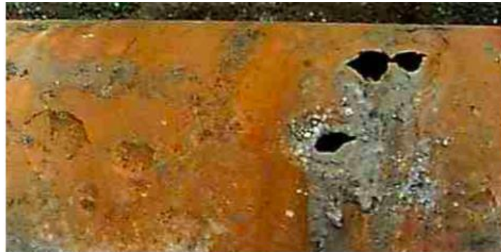
Figure 2-35: External corrosion of ductile iron pipe
