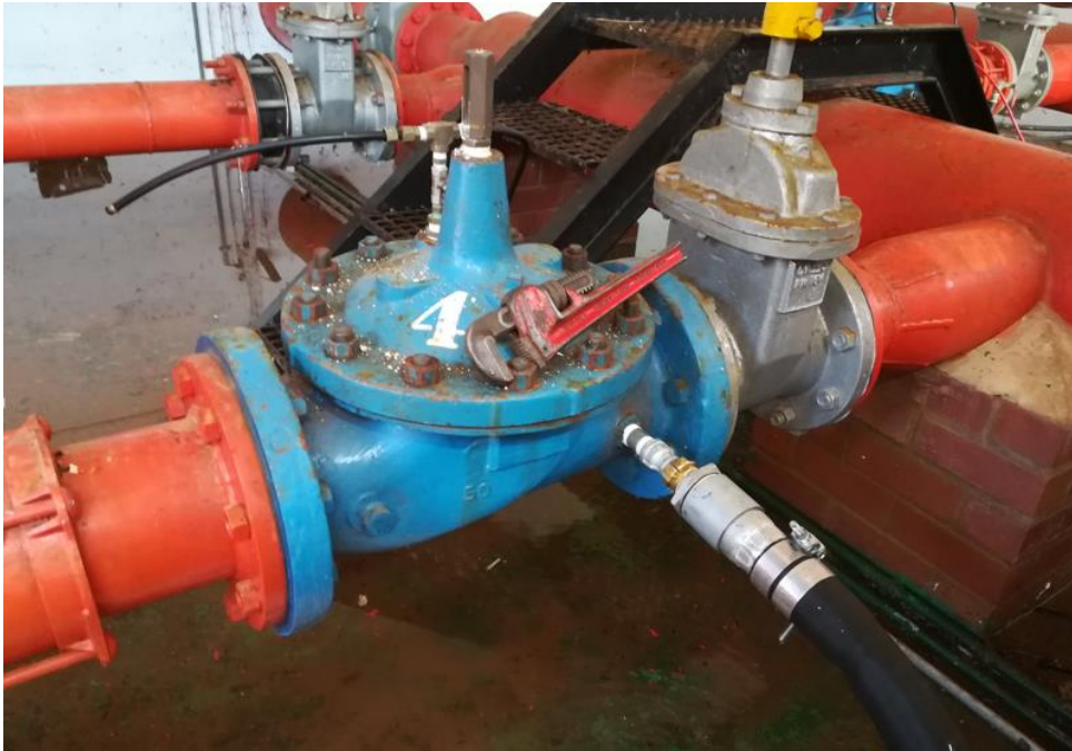
Figure 5-38: PCAE connection point on the PRV
