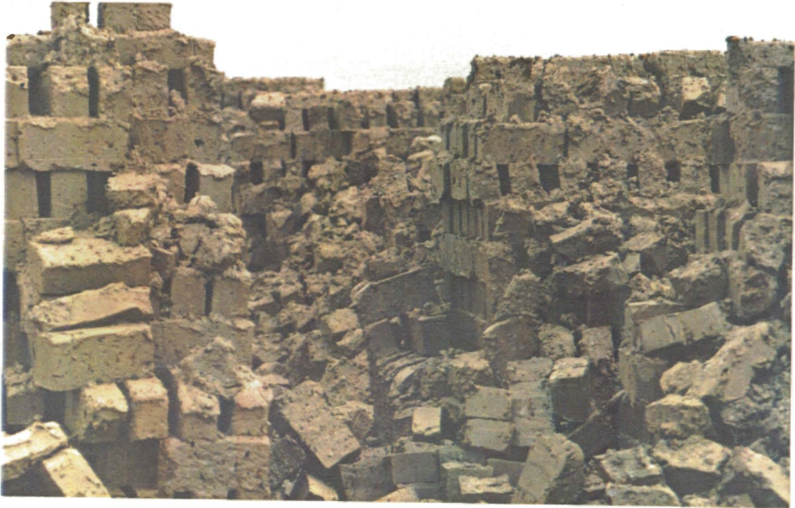
Rain damaged square pallets at Joostenberg Brick April 1993.
