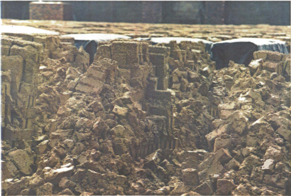
Rain damaged square pallets at Joostenberg Brick April 1993
