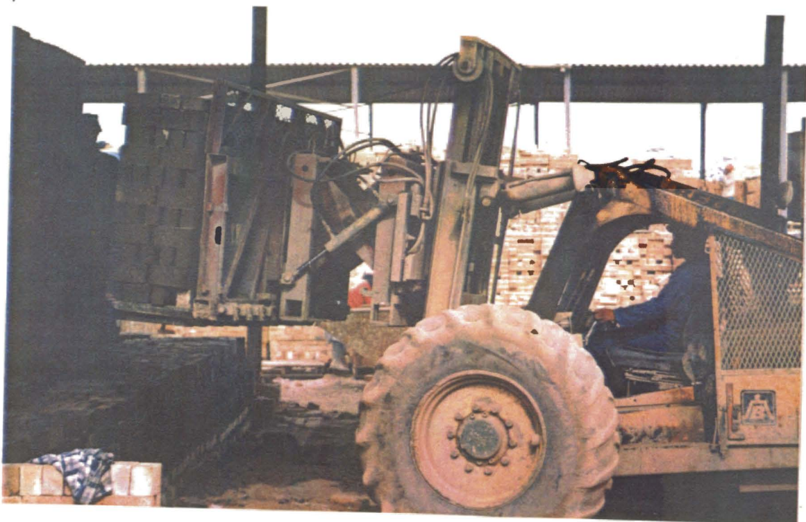
The hydraulic mechanism is being extended to position the stack of bricks.
