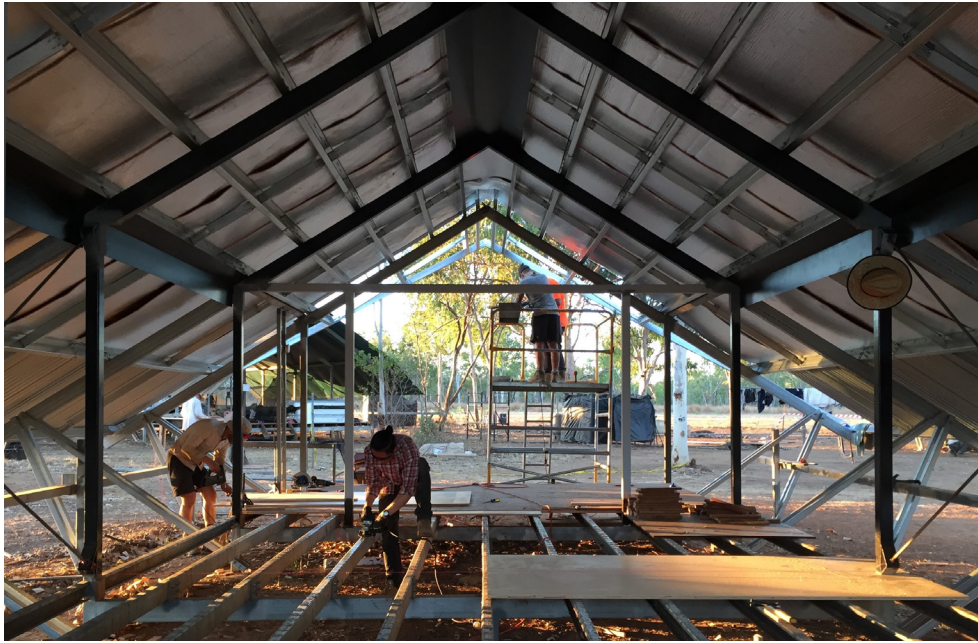
Figure 8: Rangers' accommodation under construction. The existing steel structure and foundations have been reused and incorporated into the new buildings. The roof has been updated with reflective insulation and a ventilated cavity to provide better protection from the sun (Joti Weijers-Coghlan 2018).
