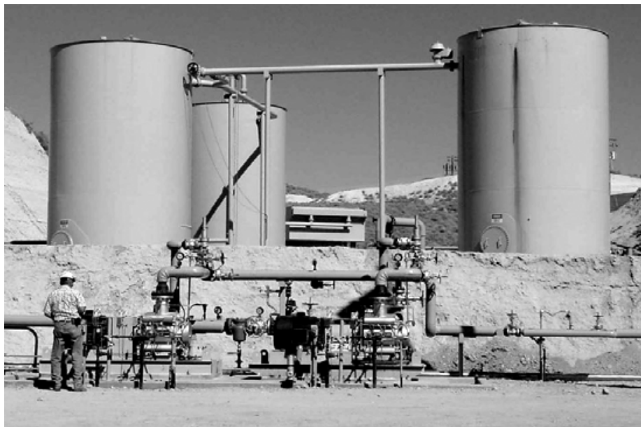
Figure 4: Separators in Oil Field
