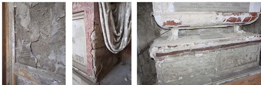
FIGURE 5 Examples of damages due to the capillary rise of water and salts in masonries of the monumental Certosa cemetery in Bologna, Italy
