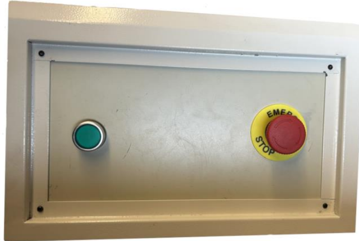
Figure 25. The face of the Control Box Installed on the Control Box
