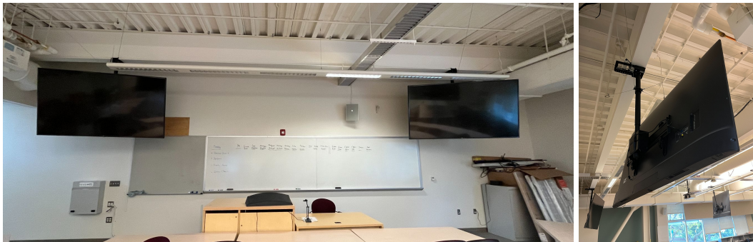
Figures 3 and 4: Ceiling-Mounted Television Screens in Room B202
