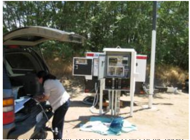
SCADA Enclosure is open in the center of the photo.
