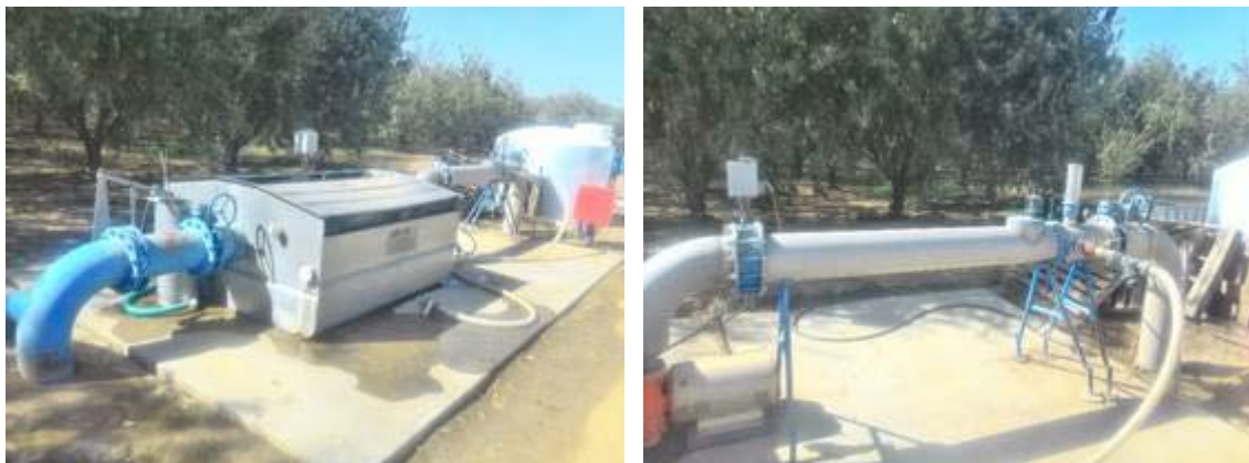
Figure 4. Filter station at Participant 4 (left) and flow meter location (right)
