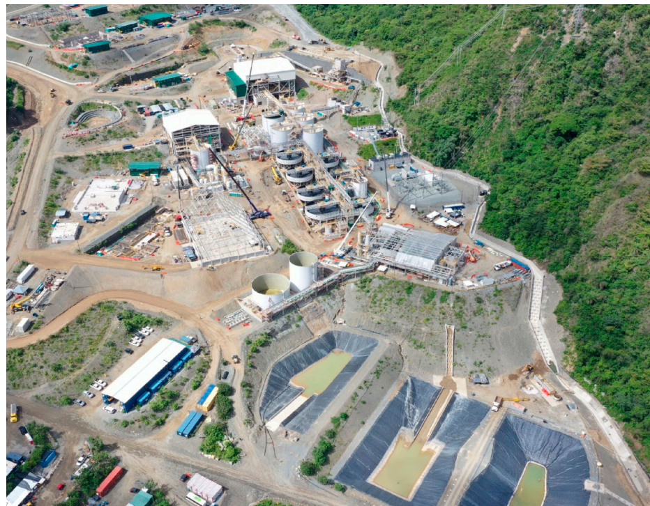
Figure 18. View of sulphide gold concentrator plant, showing gravity concentration, cyanide leaching, counter-current decantation (CCD) thickening, and Merrill Crowe processes.
