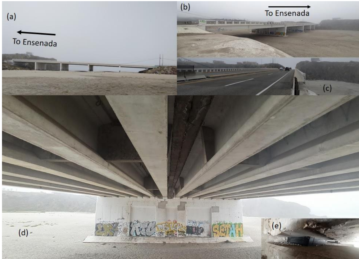
Figure 2: La Mission Bridge. (a), (b) and (c) Road view, (d) pier view and (e) neoprene plates.
