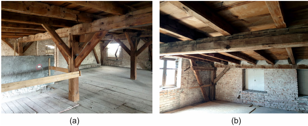
Figure 2: Photographs of the roof framework from the Monastery of Congregation of the Sisters of St. Catherine in Orneta (Poland).
