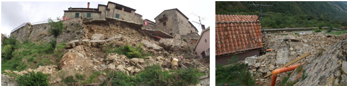
Figure 3: Collapse of the city walls in Cana di Roccalbegna (October 5, 2013). On the left: the collapse seen from below; on the right: the debris near the building below the wall.
