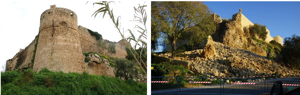
Figure 2: The collapse of city walls of Magliano in Toscana (November 13, 2012). On the left: the “Torrione” before the consolidation; on the right: the “Torrione” after the failure.
