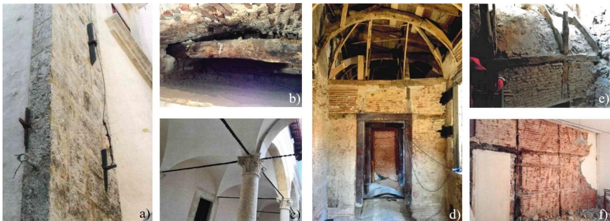
Figure 7: Anti-seismic measures adopted in Carli Benedetti Palace in L'Aquila: a) heads of the metal tie rods connecting vertical walls to horizontal structures; b) timber (radiciamento) reinforcing a masonry wall, connected to a metal tie rods crossing a chimney flow; c) tie rods at the intrados of the arches of the porch; d) the 18 th century additions composed by wooden frames, directly connected to e) the wooden reinforcements of the vaults, forming a box-like devise with f) the vertical partitions (pictures from [15] elaborated by the authors).
