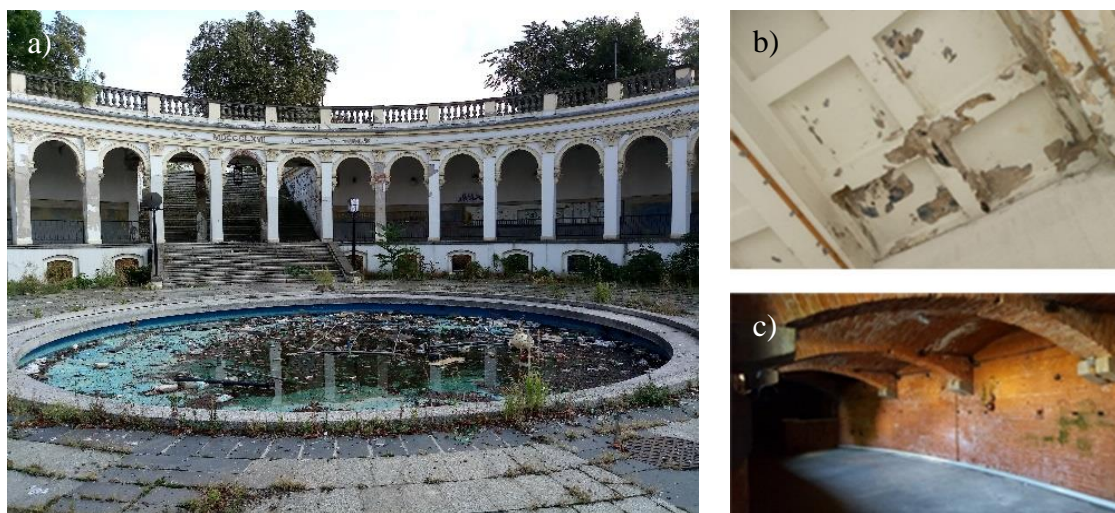
Figure 3: General view: a) the colonnade building (in the foreground is a swimming pool with a fountain); b) the slab-ribbed reinforced concrete ceiling; c) the basements and the brick ceiling
