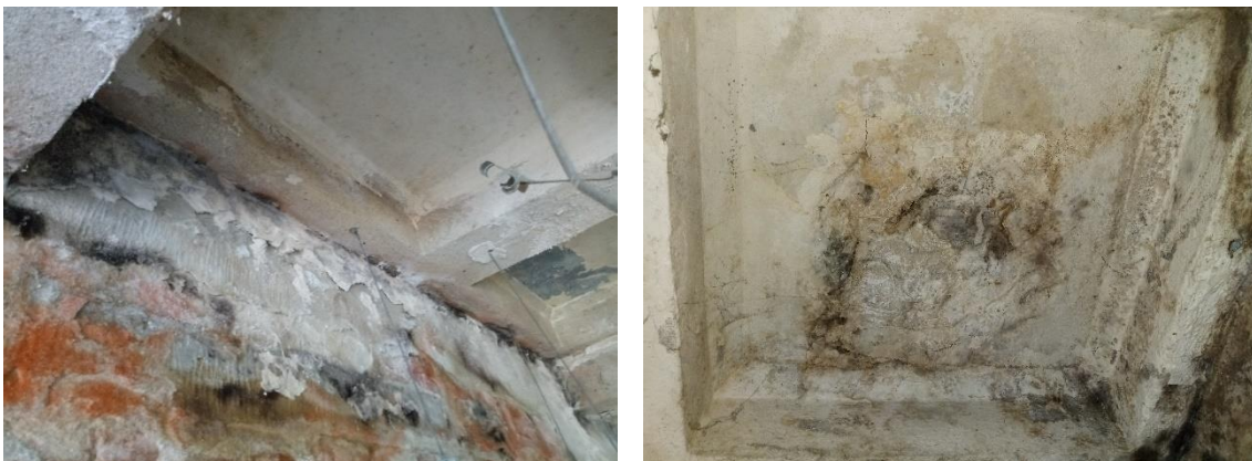
Figure 9: Sample view of moisture and patches of corrosion of a reinforced concrete ceiling
