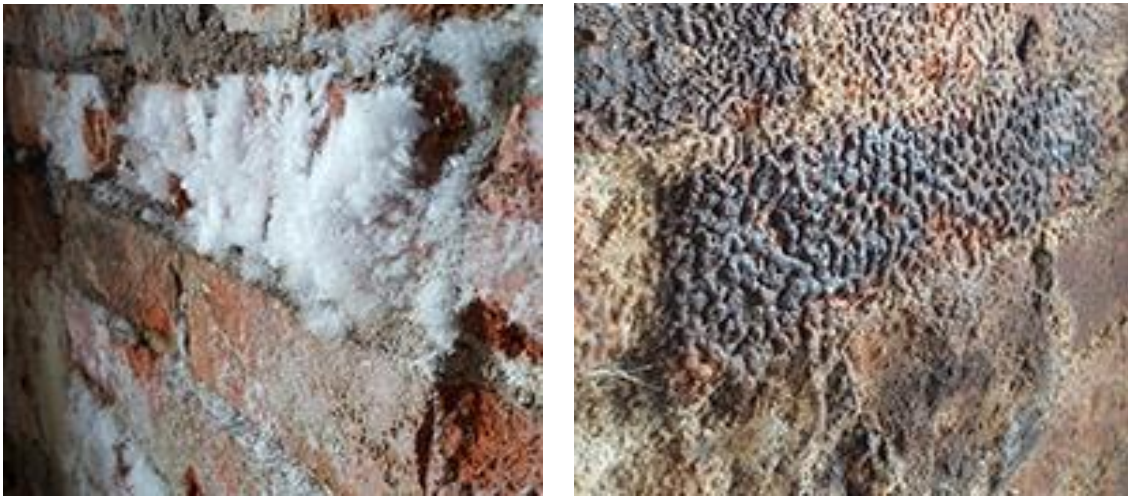
Figure 8: View of a fragment of a brick wall that is very wet and covered with mold fungi
