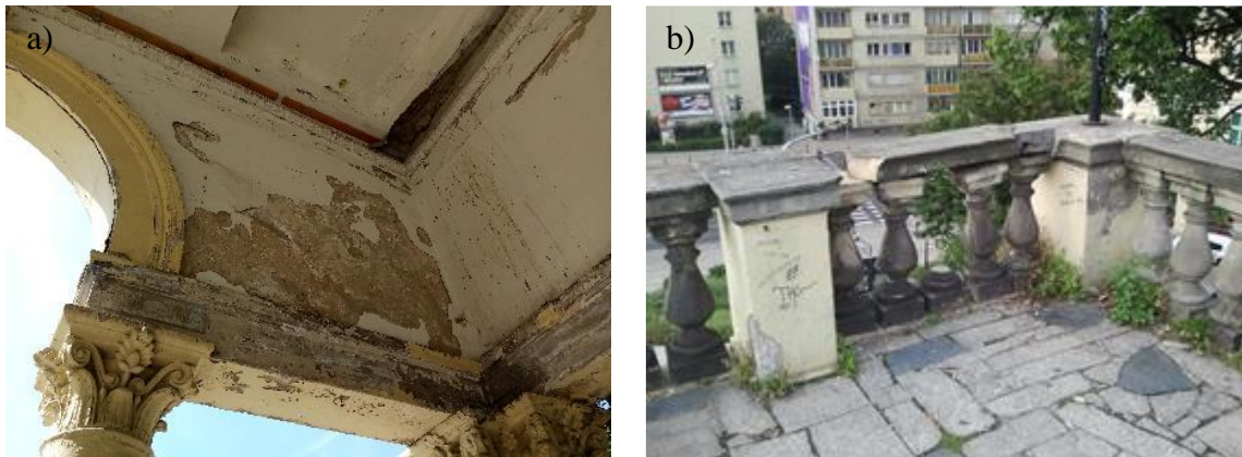
Figure 4: View: a) damage to stucco and plasters in the colonnade building; b) incomplete elements of the balustrade and granite floor
