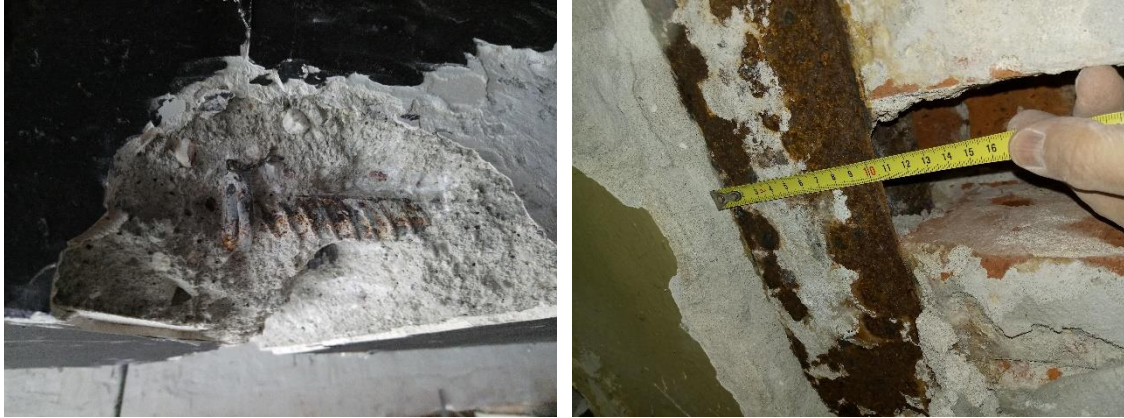
Figure 11: Exemplary view of: a) reinforcement in a reinforced concrete girder; b) flat bottom rail's foot
