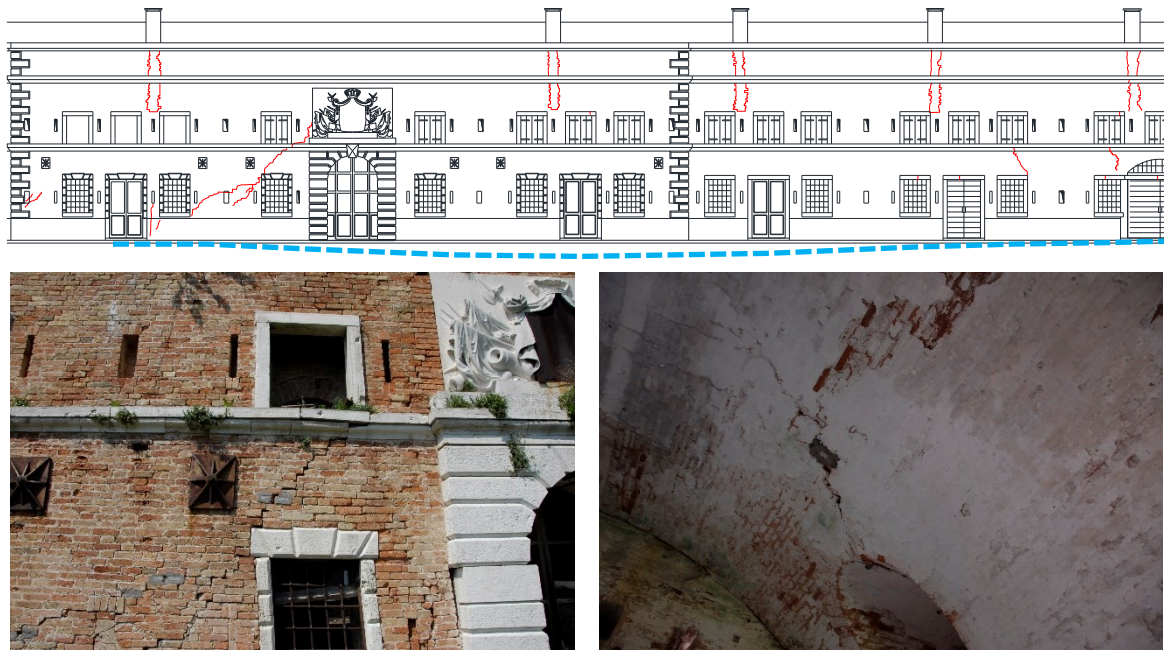
Figure 5: crack pattern in building nr. 8: it is highly visible a well-defined differential settlements trend
