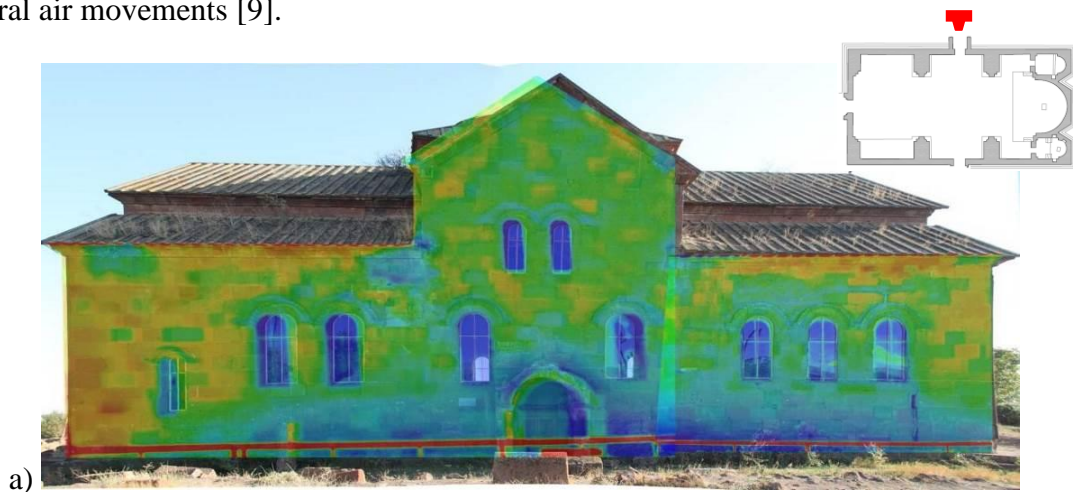
Figure 4a: The thermography test investigations, conducted on the North front external side.
