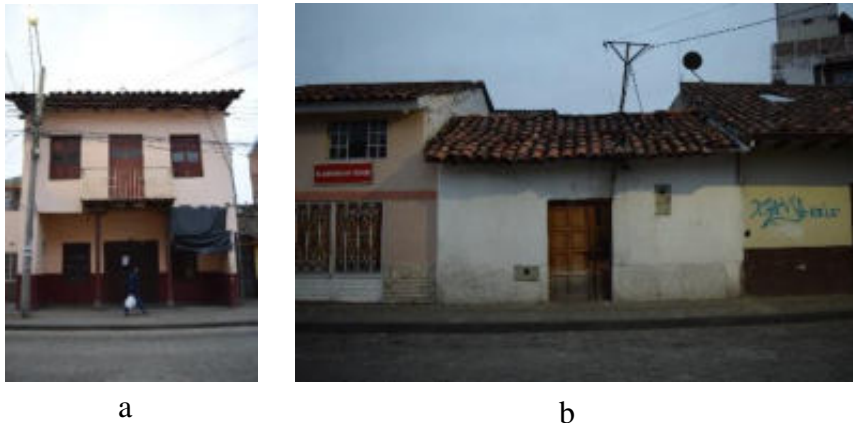
Figure 6: Buildings with threats because of electrical installations: a) E204, b) E107 and c) O206 Source: a, b) Photographical archive of the World City Heritage Project, 2018
