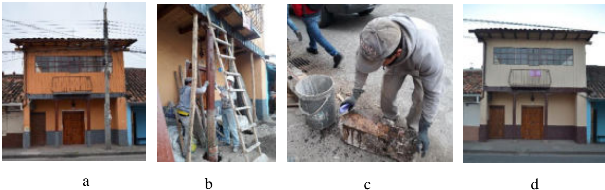
Figure 5: León House (E204); main facade before the intervention; b) showing of the portal during the replacement of the bases; c) original unburied bases; d) columns after the intervention Source: a, b,c,d) Photographical archive of the World City Heritage Project, 2018
