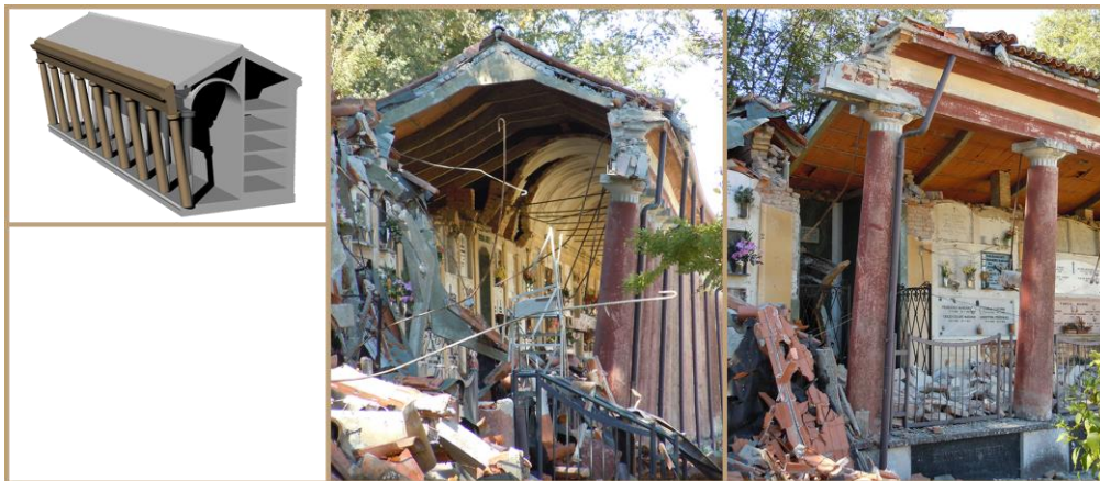
Figure 4: Cemetery of Mirandola - Tipping over away from the colonnade floor. It is worth mentioning the use of reinforced concrete beams and elements in steel in the structures.
