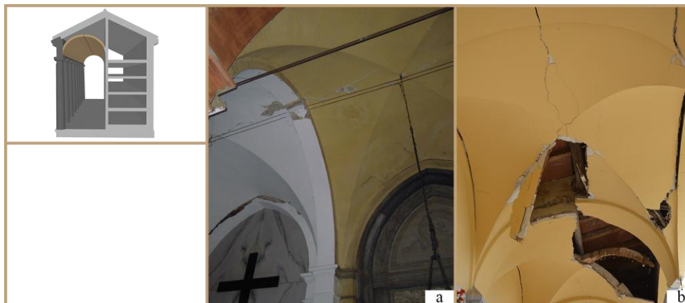
Figure 5: Cemetery of Bondeno (a) and cemetery of Mirabello - damage to the vaults
