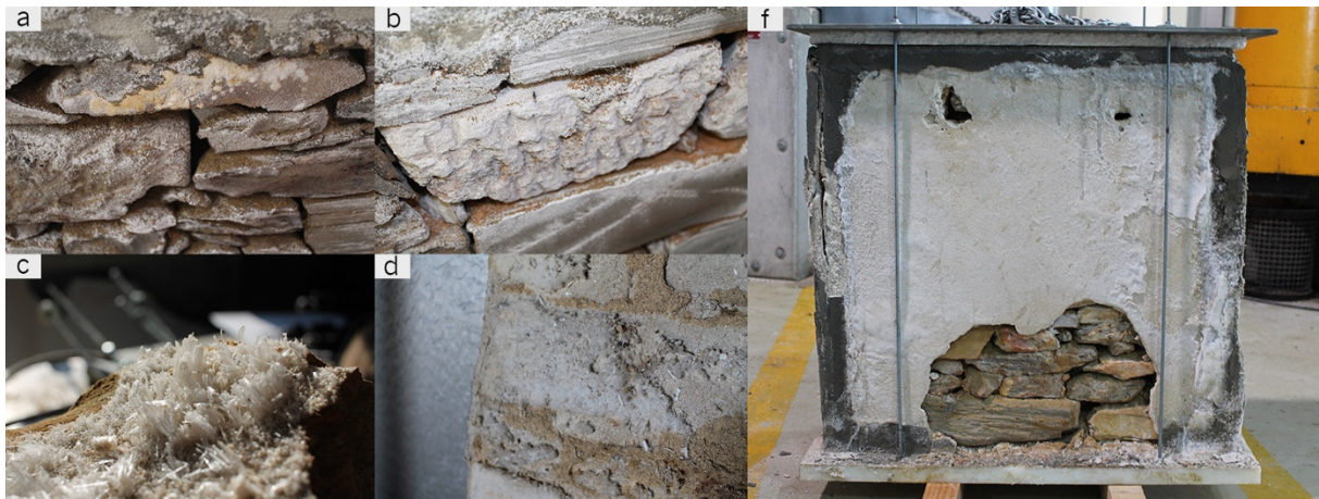
Figure 6: Damage observed during the WA test: (a) and (b) examples of different salt deposits on schist stone; (c) efflorescence; (d) efflorescence located at the coating/masonry interface; (f) example of WAC with superficial salt deposits, ruptured lime coating and detached lateral covers.
