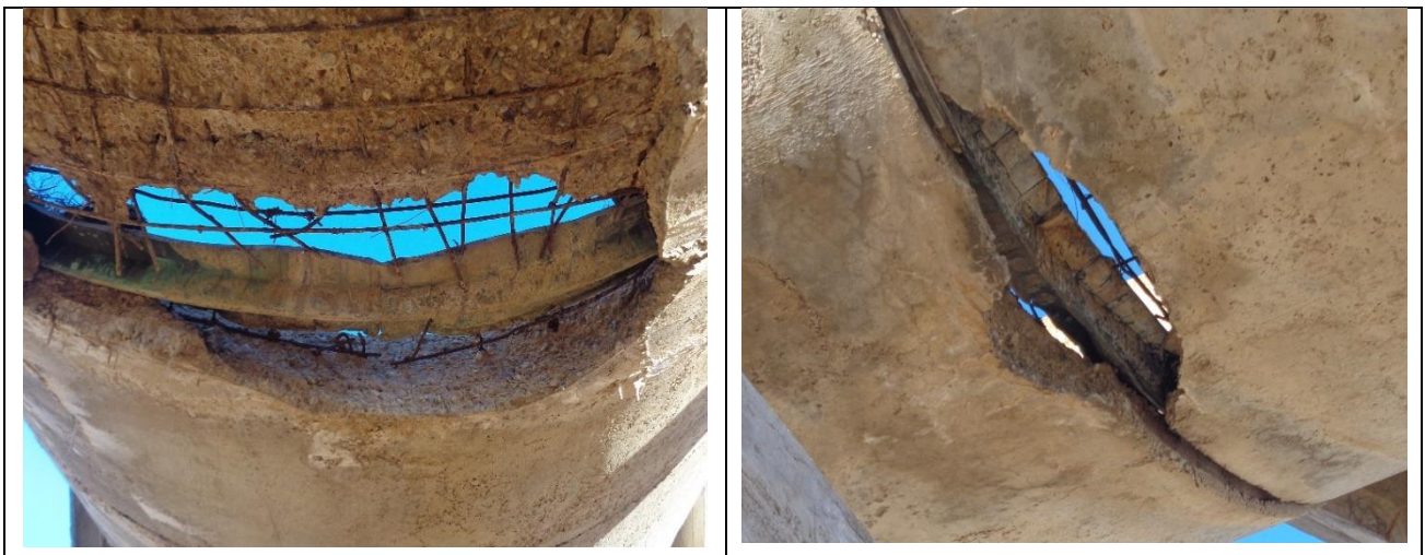
Figure 11 : Deterioration of flume at expansion joints
