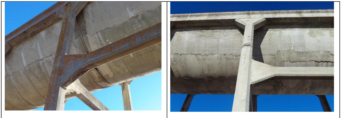
Figure 8 : Lichen on a column and beams on the north side of the aqueduct (left) due to the existence of more humidity and cooler temperatures compared the south side (right)
