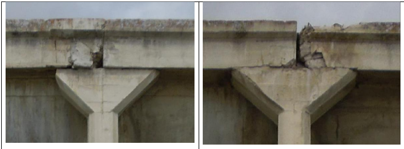
Figure 13 : Deterioration of longitudinal beams near expansion joints
