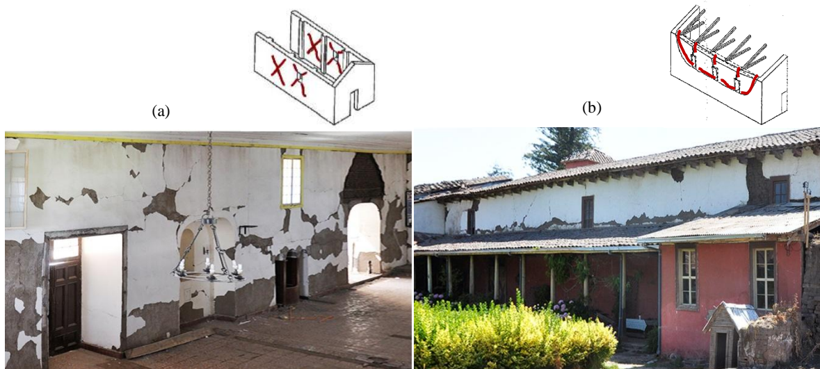
Figure 4: Deep cracks observable in the (a) internal and (b) external elevations of side walls [5]
