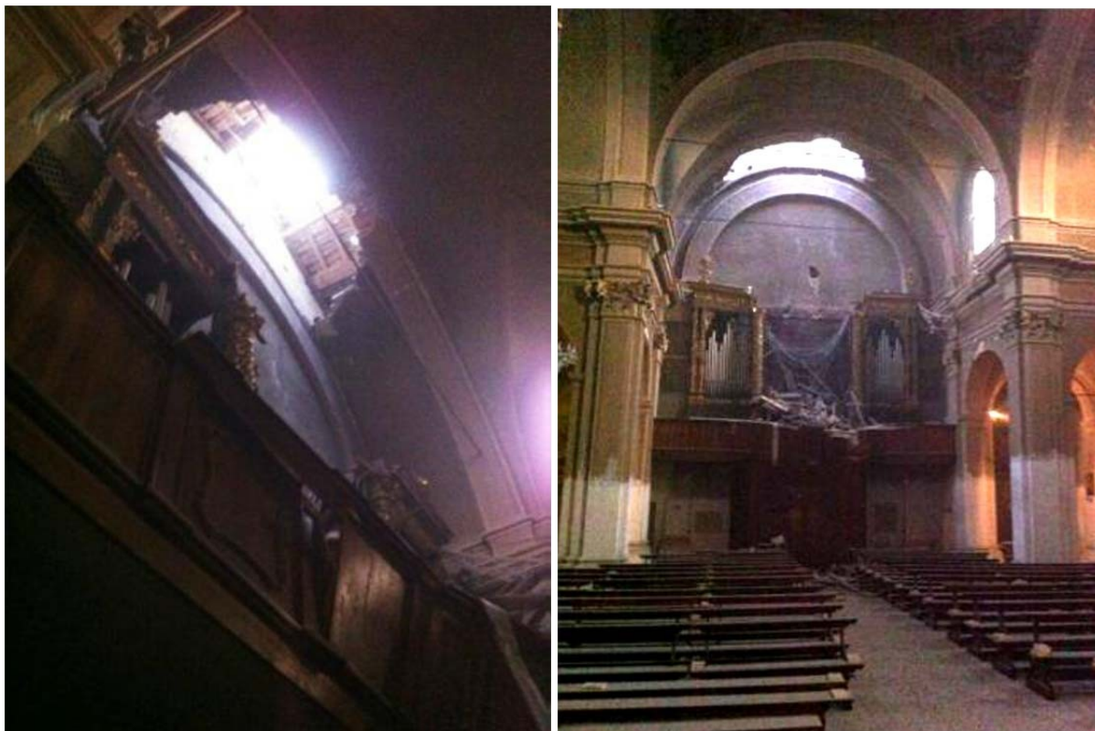
Figure 5: Collapse of the vault behind the façade
