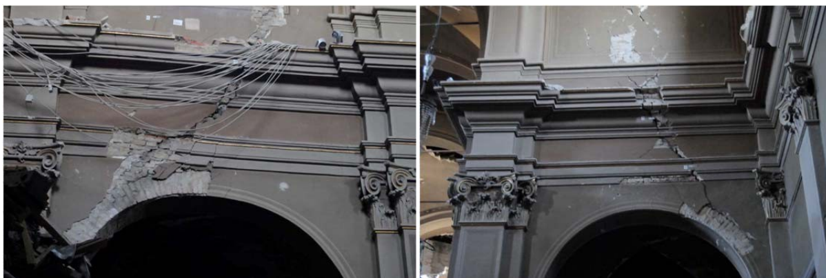
Figure 6: Cracks in the arches along the nave and transversal to it.
