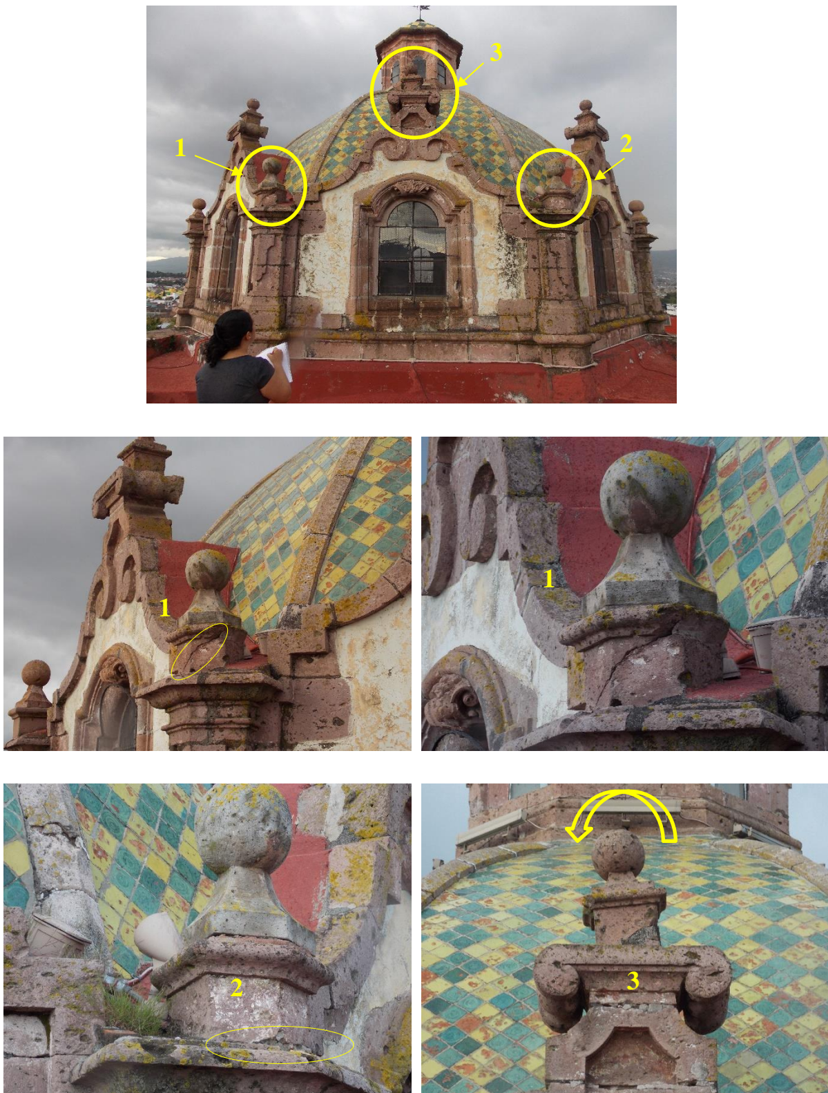
Figure 8: Pinacles rocking and shear base damages
