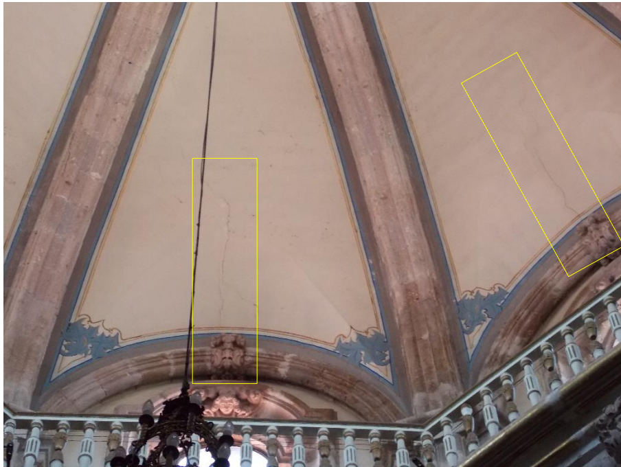
Figure 7: Cracks on the masonry dome
