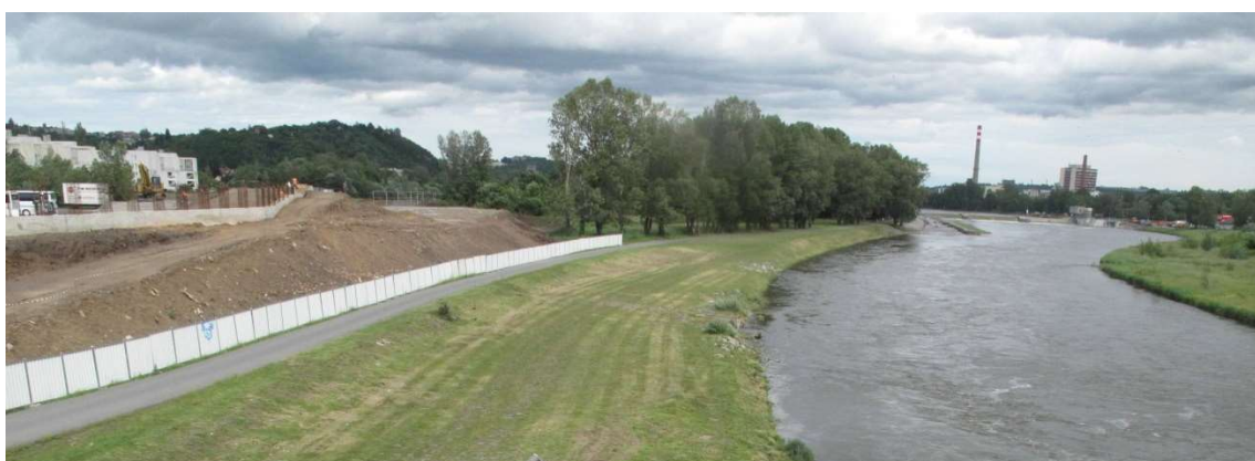
Figure 2: Construction phase of the combined earth levee, permanent reinforced concrete wall with columns prepared for temporary metal barriers.
