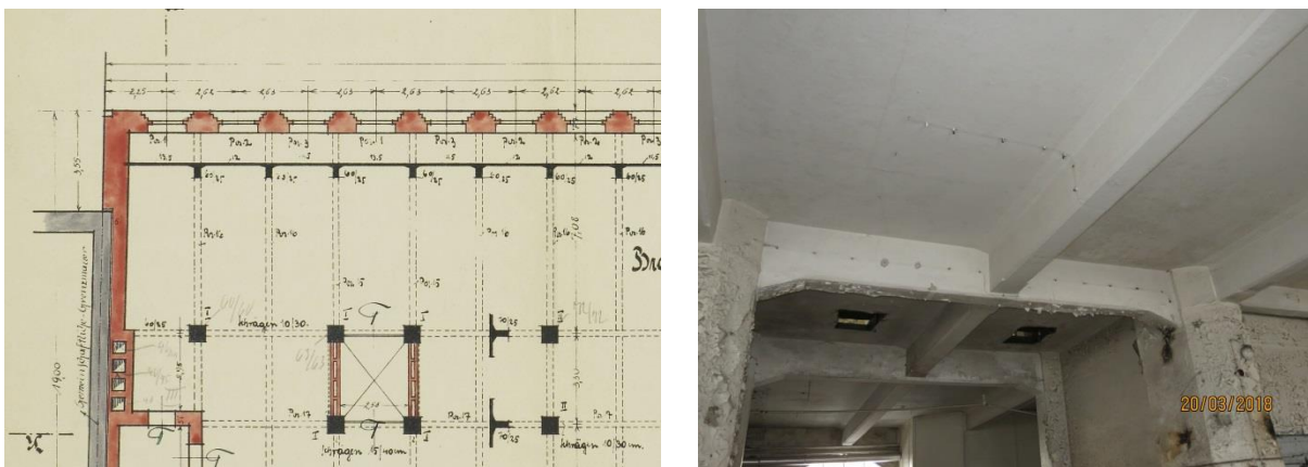
Figure 8: Archival drawing and general view of the RC rib floor in a bakery plant (1913)
