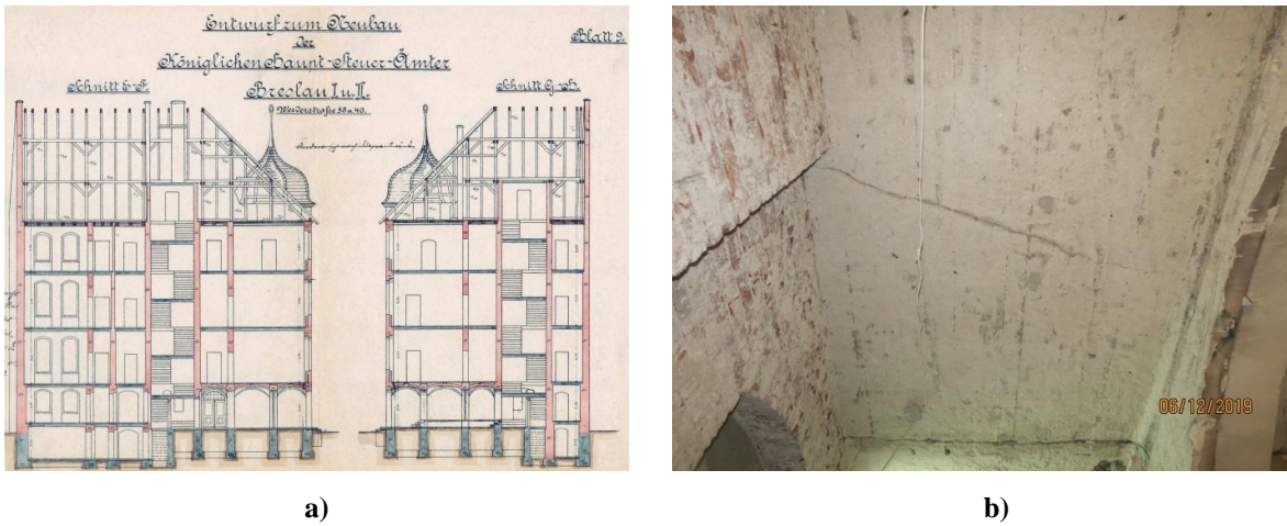
Figure 11: a) Archival drawing of building cross-section; b) typical cracks in floor slabs
