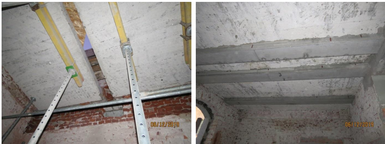
Figure 13: a) Floor slab with cuttings; b) floor with additional inverted T-shape RC girder supports
