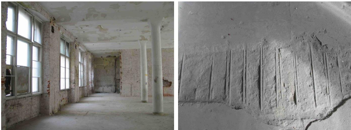
Figure 5: General view and rebar exposure of Koenen plate floor in a public service building
