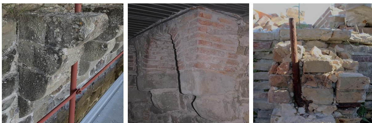
Figure 6: From the left: stone cantilevers in the corbels of eastern curtain wall; stone cantilevers supporting brick arches; I-beam with L shaped anchor bar in one of the brick masonry corbels of the polygonal tower.
