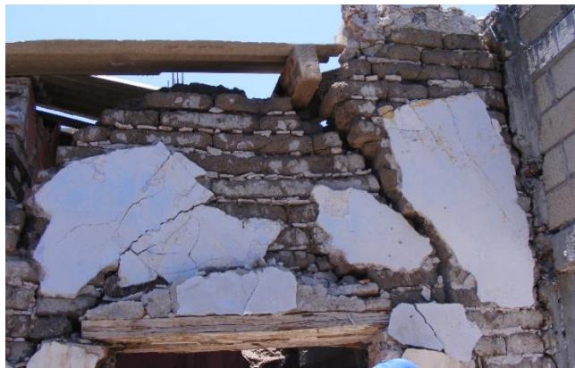
Figure 3: Damaged adobe building with mixed construction techniques
