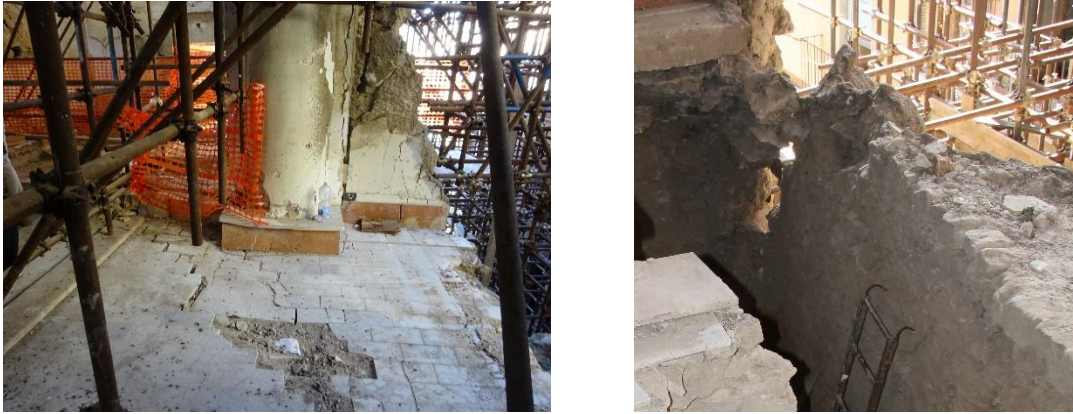
Figure 2: Crack on the floor in proximity of the pillar and the rotation of the wall under the collapsed one
