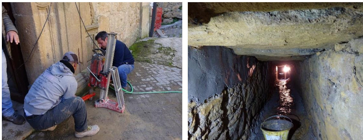
Figure 7: Perforation in the ground and interior view of the conduct
