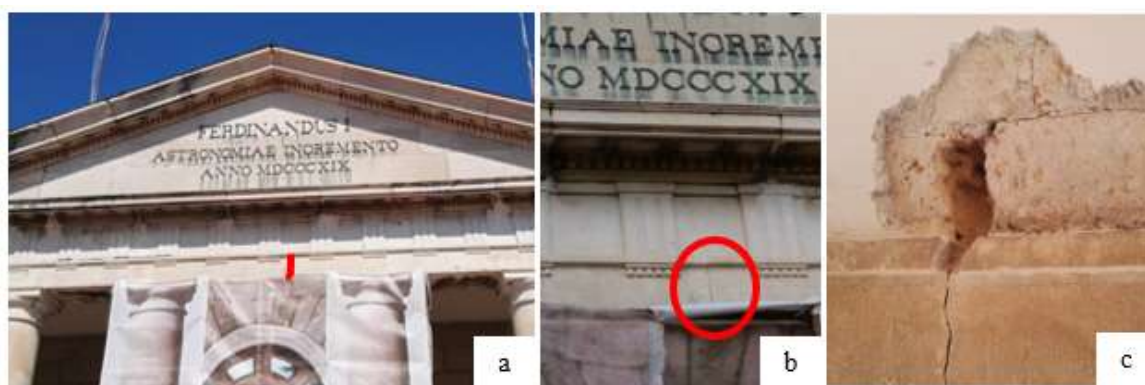
Figure 15: Crack at the midspan of the stone lintel (a-b); c) essay at the internal side.
