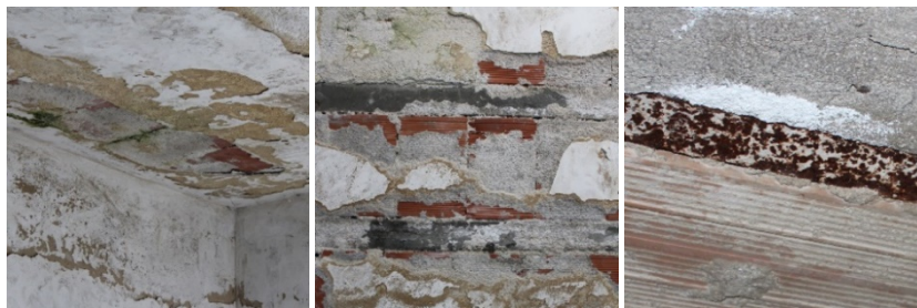
Figure 7: Accelerated degradation of structures due to the design errors illustrated in the text
