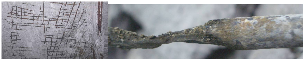
Figure 3: Typical rebar corrosion: a) lower side of a slab (structure Nr 5) b) detail of pitting (structure Nr 4)
