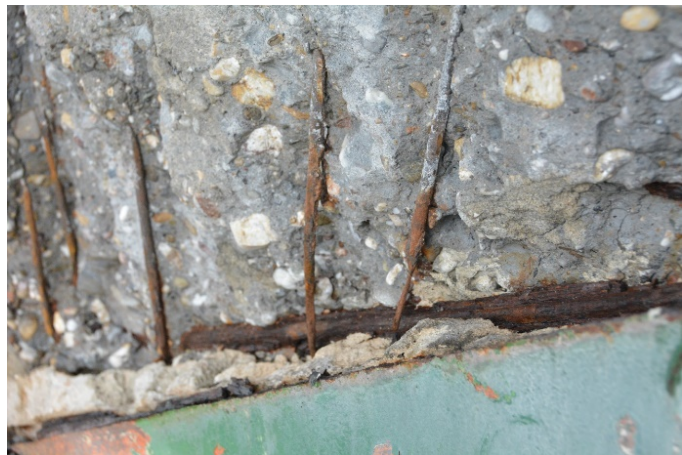
Figure 1. Loss of rebar section due to corrosion in exposed concrete beam from 1921
