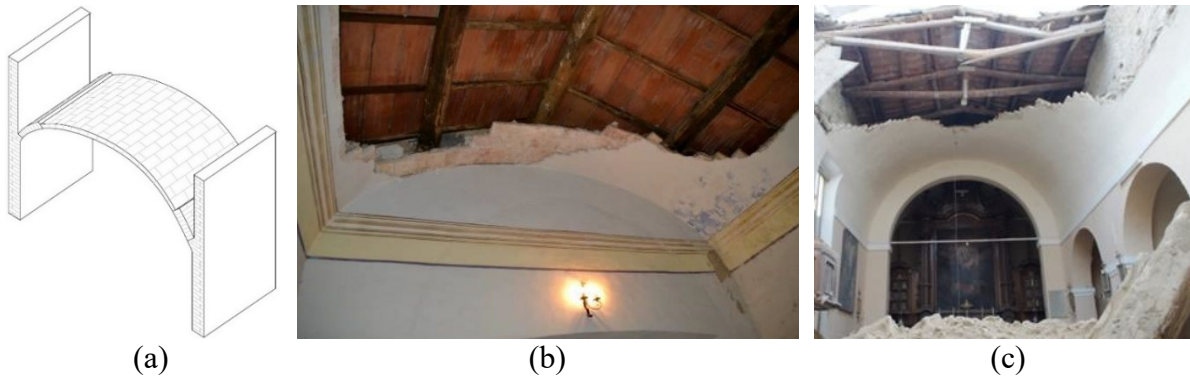
Figure 1: Brick in folio masonry vaults: (a) typical configuration and examples of vault failure occurred (b) in the St. Egidio's Church of Guardea, Italy [2] and (c) in the Capuchins' Church of Urbino, Italy (ifg.uniurb.it)
