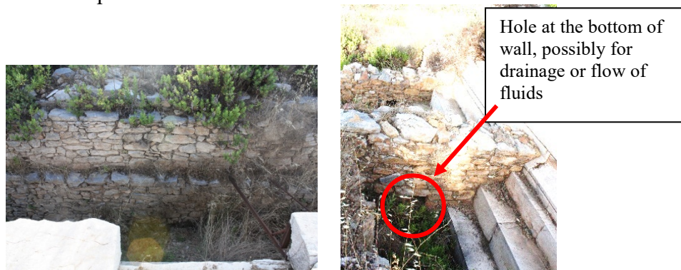
Figure 2. (a) The retaining wall on the north side, (b) One of the perpendicular walls with bottom hole on the east side
