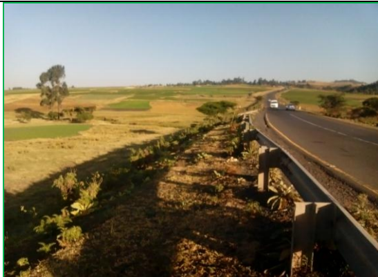
Fig 3.8: Wacan Mazoriya Existing Road Condition.
