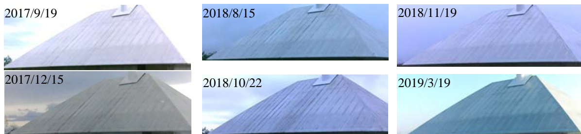
Figure 4. Photographs of NE roof from September 2017 to March 2019.
