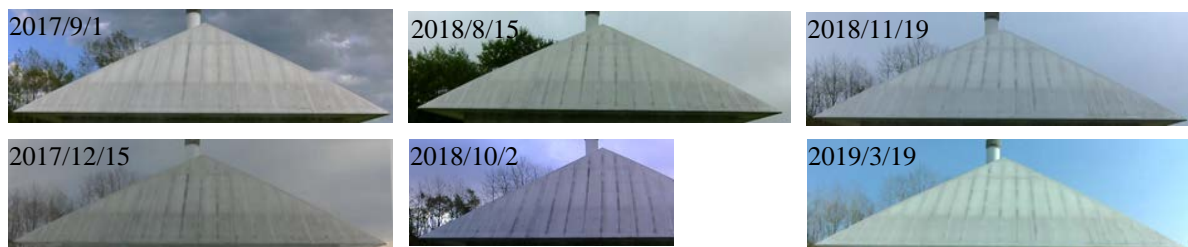
Figure 5. Photographs of NW roof from September 2017 to February 2019.
