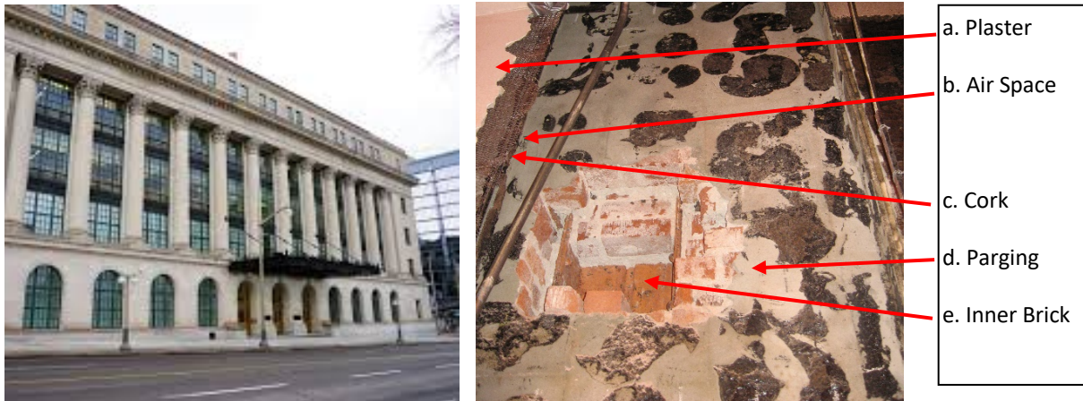
Figure 1. General elevation view and cross section of exterior wall showing parging and interior red brick behind Indiana limestone veneer. Black spots are mastic used to bond one-inch cork insulation (Interior photo courtesy of JM Carriere of Adjeleian Allen Rubeli Ltd.).
