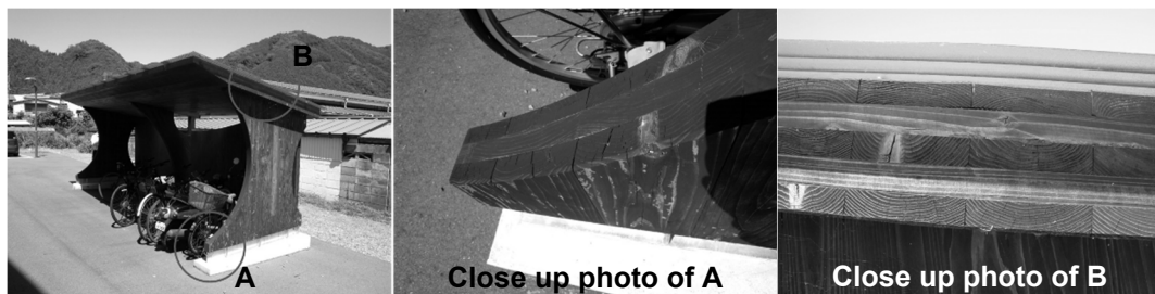
Figure 1. Deformation of CLT exposed to outdoor climate (Bicycle parking space).
