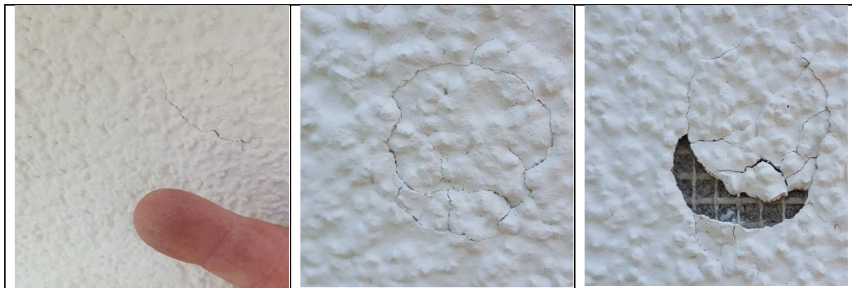
Figure 3. Representations of the damage classes: crack (left), full circle fracture (center) and breakout (right).
