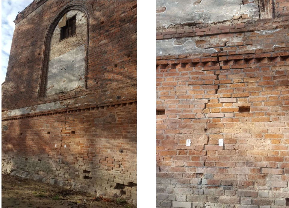
Figure. 4 Slanting church wall.
