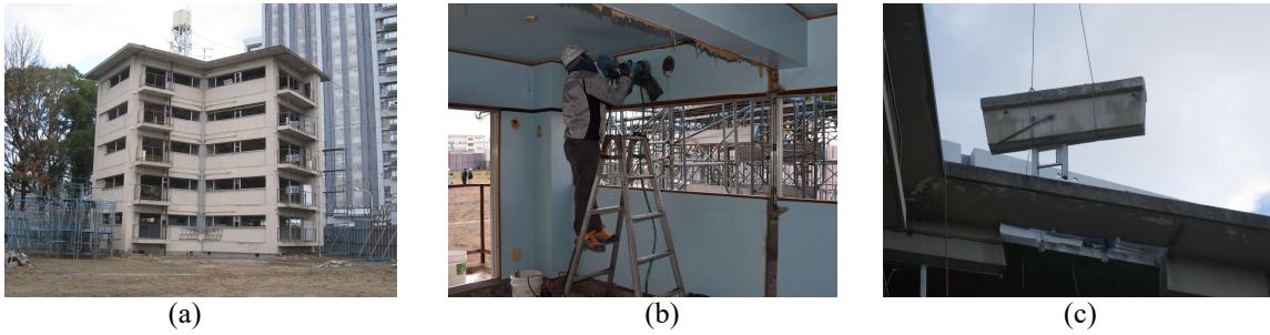
Figure 1. Existing building (a) comprehensive view of the test building; (b) concrete core boring; (c) cutting girder with a wire saw.
