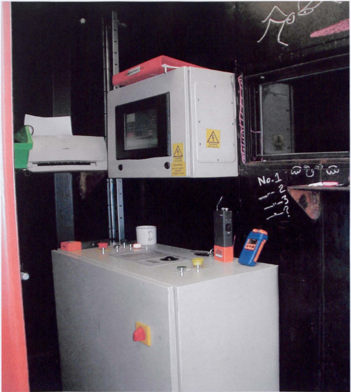
Figure 1.3 – Control room of the FFU.
