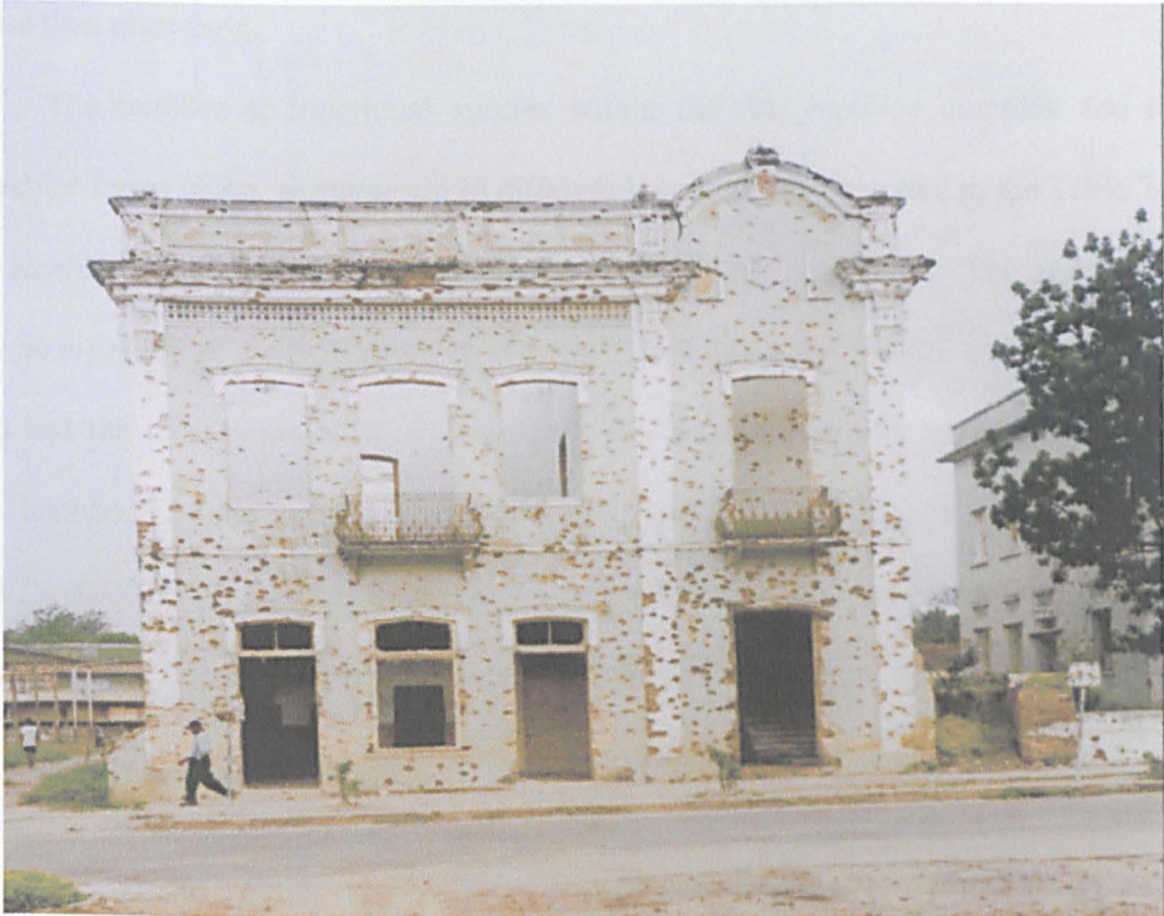
FIGURE 7.3. Huambo: A stunning colonial style building destroyed by the war. Huambo now lies in ruins and has one of the most concentrations of land mines in Angola. Huambo was at the epicenter of the civil war and almost every building has been scarred by bullets and shells (Paulo Kassoma, Huambo's Governor, http://www.washingtonpost.com/wp-adv/specialsales/spotlight/angola/article19.html ).
