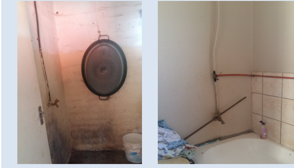
Photo 12: Plumbing problems in the RDP house, Cosmo City township. Source: Fieldwork, 2017
