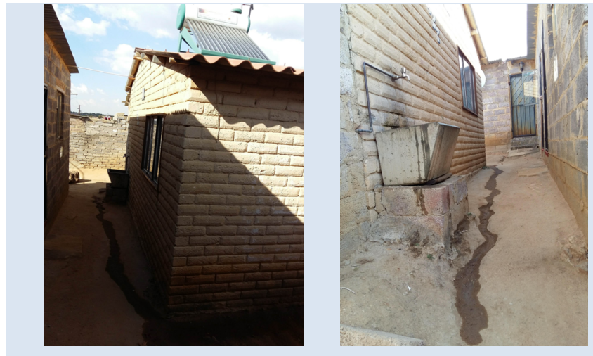
Photo 13: Leakage from the SWHs, Cosmo City township. Source: Fieldwork, 2017
