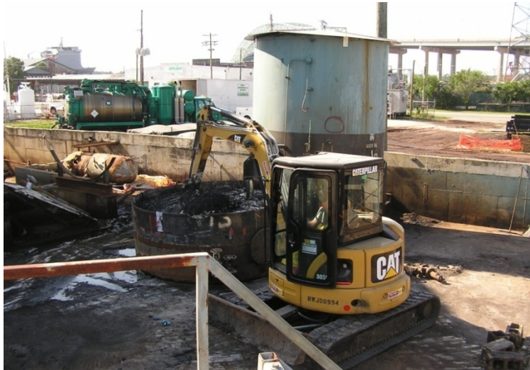
Figure 5. Treatment of sludge in small tank
