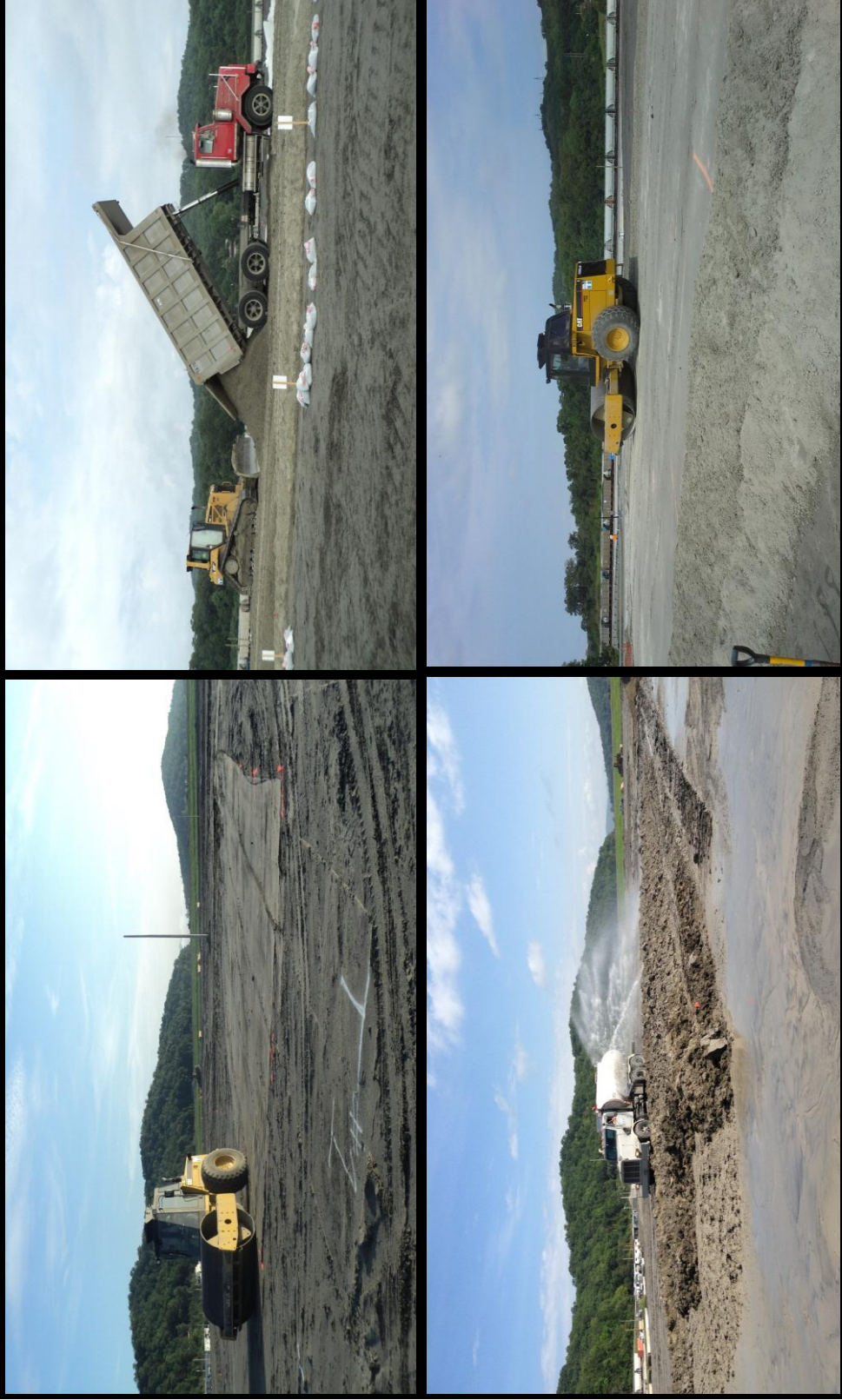
Figure 2. Test Pad General Construction Process (from top left: subgrade preparation, fly ash placement, moisture conditioning, and compaction)
