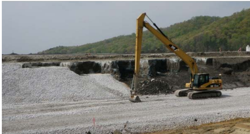
Figure 10. Excavation of ash between completed slurry walls and placement of the rock berm along the restored lake shoreline.
